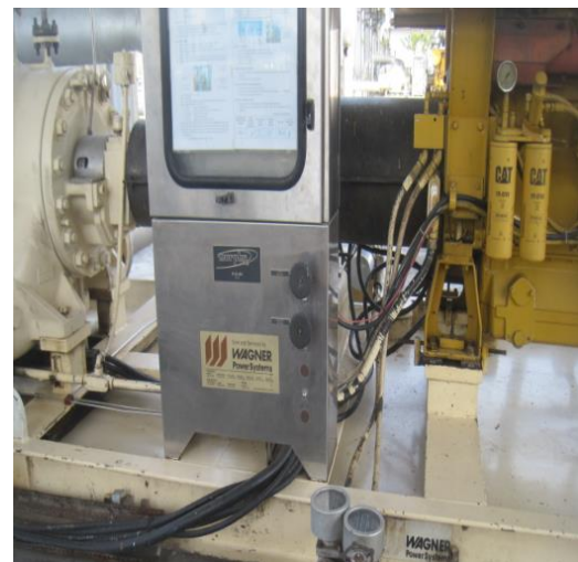
Gambar 2. Mesin Main Booster Pump Jalur 1
